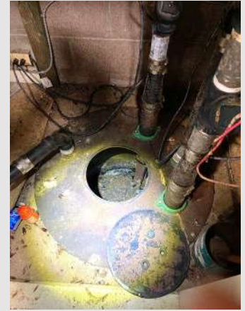
Underground Sump pump
