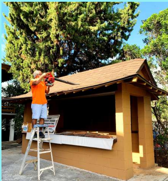
Mahalo Art for keeping the shrine debris free
